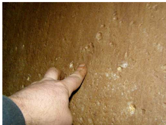
Interior shell pitting 2
