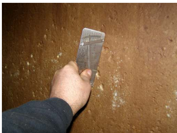
Interior shell pitting 3
