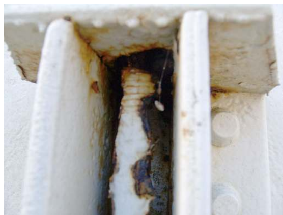
Exterior anchor bolt 5
