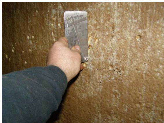
Interior shell pitting 1
