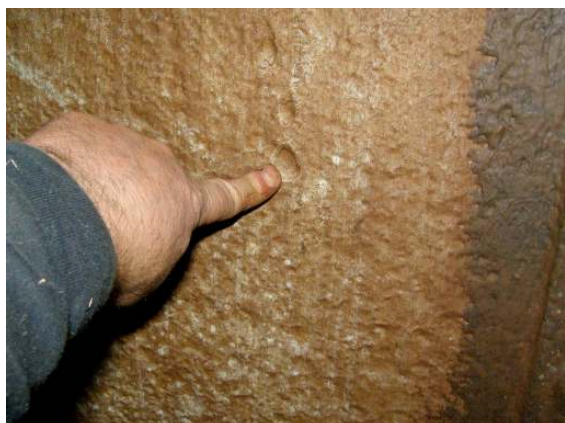
Interior shell pitting 5
