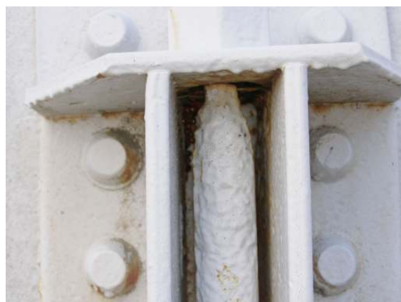
Exterior anchor bolt 15
