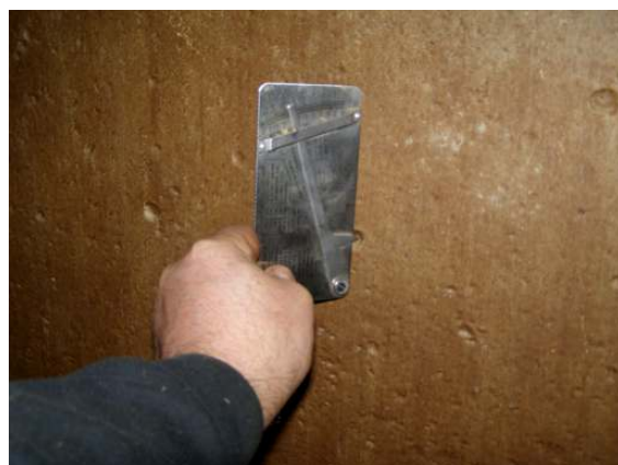
Interior shell pitting 4
